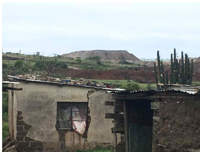
Figure 19: A damaged and cracked housing structure
